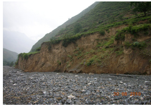
PHOTO 1. A collapse at the study area
