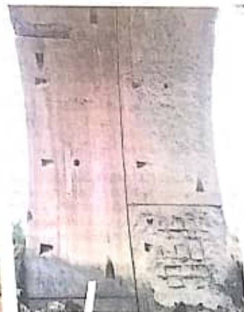
The segment with the patented concrete mixture on the left was not damaged as compared to the segment on the right that used conventional concrete for building tunnels.
