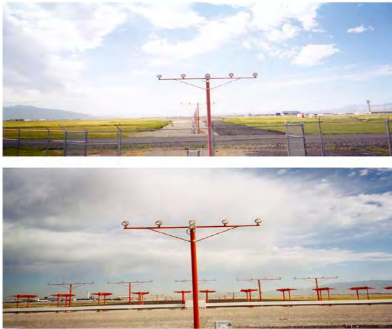
Gambar 9.1-5: Approach lighting towers — fibreglass tubular poles
