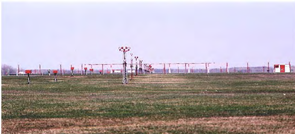
Gambar 9.1-6: Approach lighting towers — aluminium lattice structures
