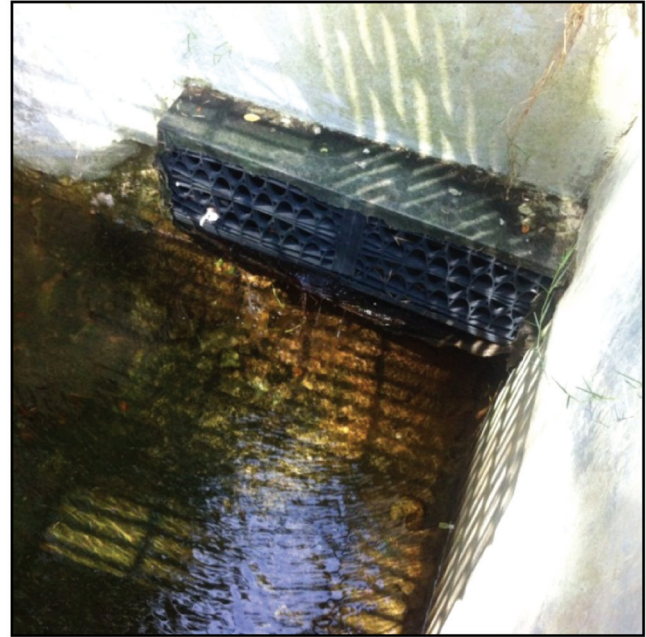
FIGURE 5. Outflow drains from swales at Astaka field
