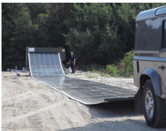
FIGURE 3. Rapid Roll is being rolled out of a trailer on site (Renovagen 2018)
