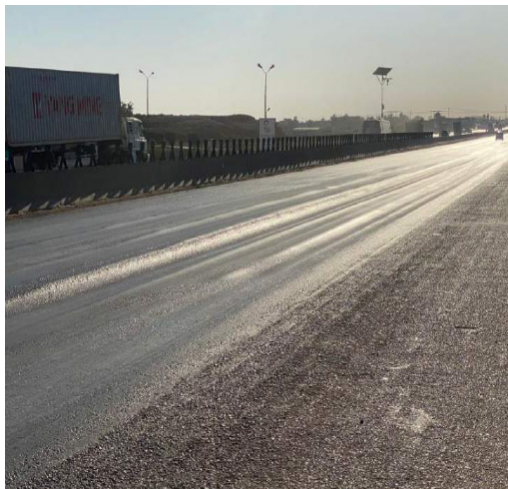
FIGURE 2. Rutting occurred in M-9 motorway due to weak subgrade soil
