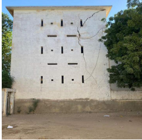
FIGURE 1. Cracks developed in MUET boys hostel due to excessive settlement
