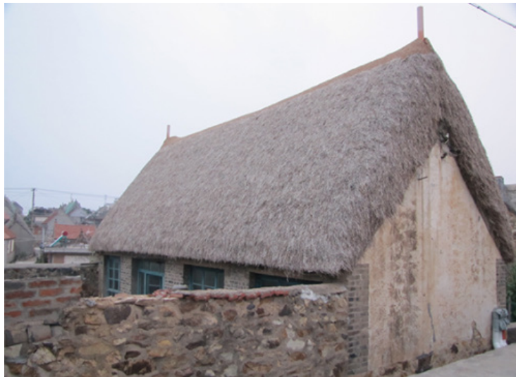
FIGURE 5. Seaweed material on roof
