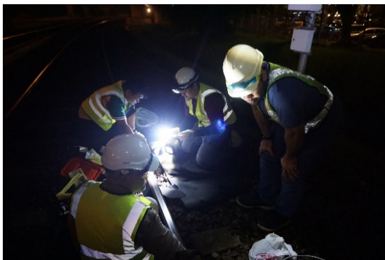
FIGURE 6. The FBG sensors installation on the railway track
