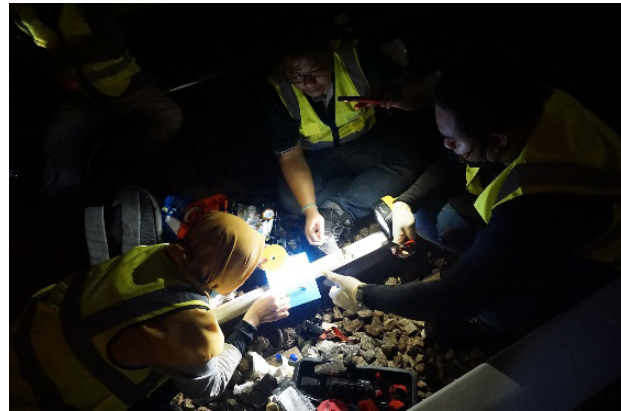
FIGURE 7. The FBG sensors are attached to the web of the railway track
