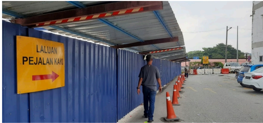
FIGURE 2. The construction site next to the transit station affects pedestrians and the scenery
