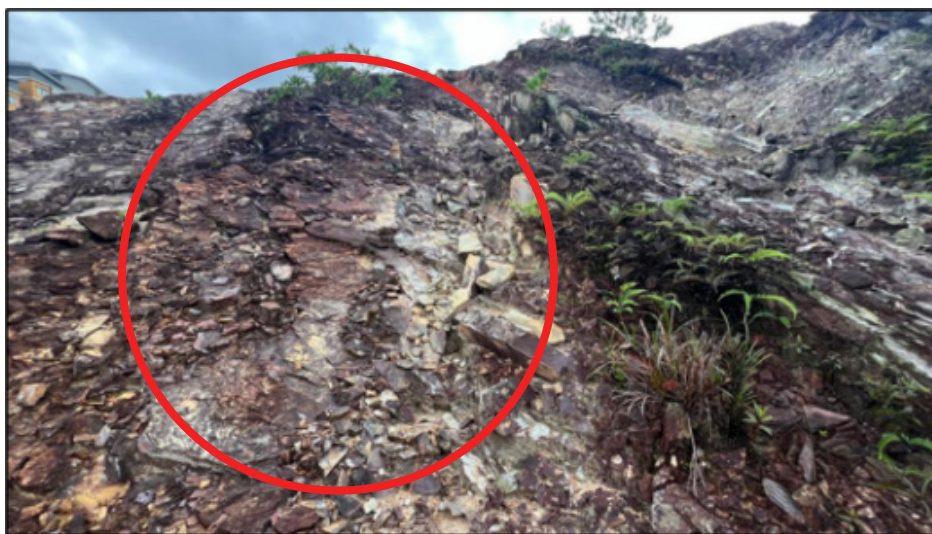
FIGURE 7. Light-coloured rock surface shows the moderately weathered condition at Location C
