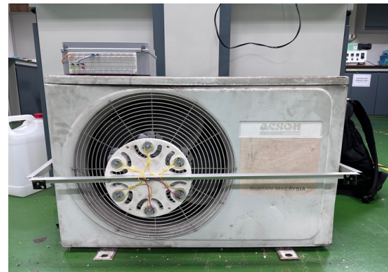
FIGURE 7. Front View of the Aircon Condenser Unit
