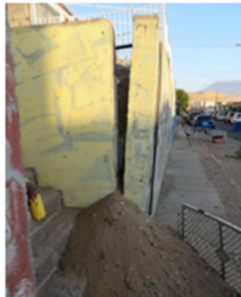
FIGURE 5. Rotation of concrete cantilever RW during the Iquique Earthquake (2014), (from Wagner & Sitar, 2016a)
