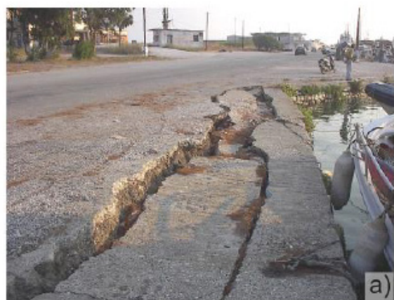
FIGURE 4. Displacement of quay RWs during Lefkada Island Earthquake (from Pitilakis & Roumelioti 2013)
