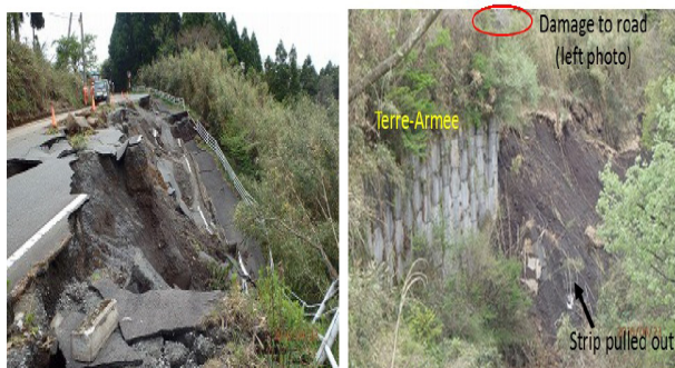
FIGURE 10. Damages of reinforced soil walls during Kumamoto Earthquake (from Kiyota et al. 2017)
