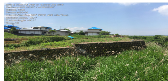
FIGURE 8. Diagonal cracks for unreinforced masonry RWs during Kumamoto Earthquake (from Kayen et al. 2016)
