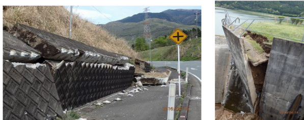
FIGURE 9. Damages of RWs during Kumamoto Earthquake (from Kiyota et al. 2017)
