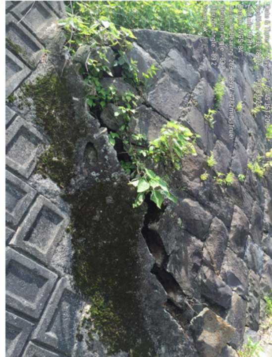
FIGURE 7. Lateral offset for unreinforced-concrete block RWs during Kumamoto Earthquake (from Kayen et al. 2016)
