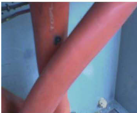
Figure 1. Example of partial discharge transform between two cable cores
