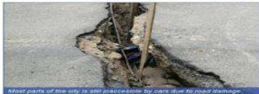
Most parts of the city is still inaccessible by cars due to road damage.
