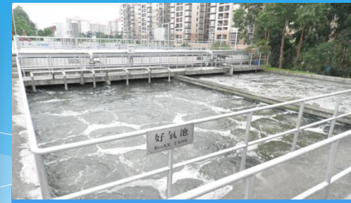
Pacific Apparel (Dongguan) Ltd - Textile wastewater Recycling (BioAX and MBR)
