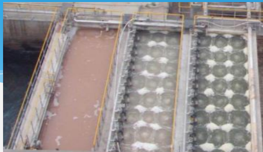
LG-DAGU Chemical Company PVC Mother Liquor Wastewater Treatment ( Recycling ) Tian jin (BioAx)
